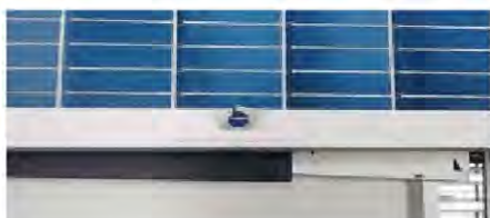
535W: torn mounting holes
