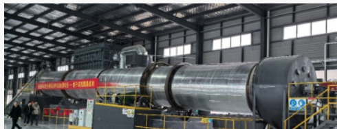
Sludge Drying System
