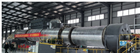
Sludge Drying System
